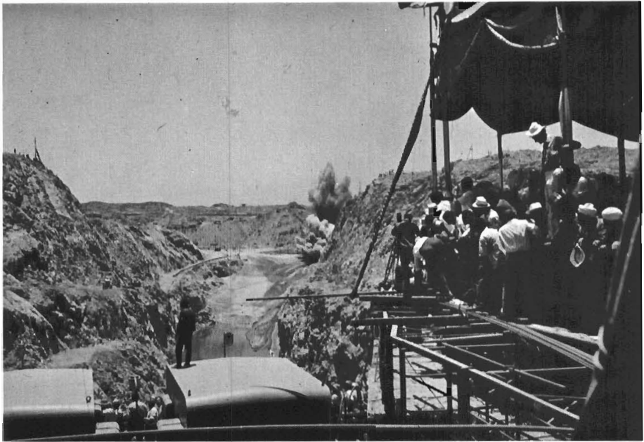
Fig. 1 — Shows the Aswan Dam when the blast was set off that diverted the Nile River.
